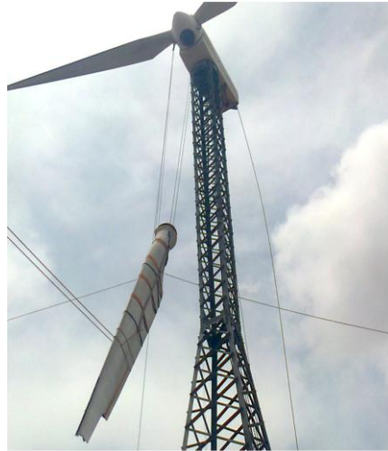
Figure 5. Damage Blade Erection
